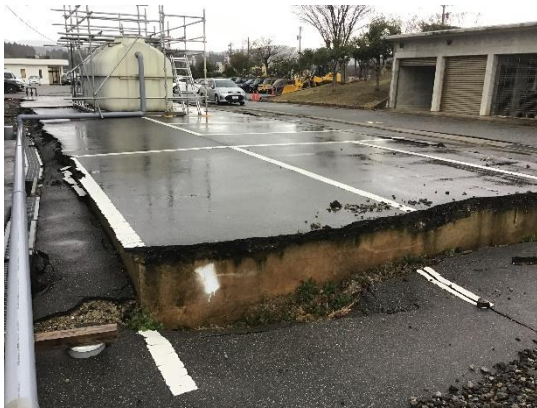
(c) 建築物周囲の地盤沈下、浄化槽
