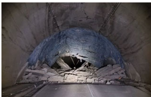
(a) 覆工の崩落
