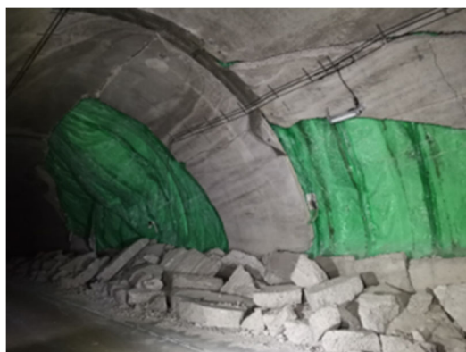
(a) 覆工の崩落
