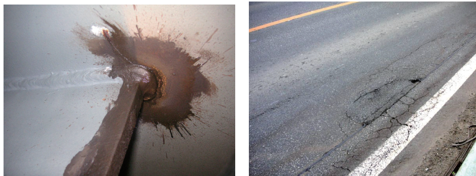
a) 鋼床版の疲労き裂
