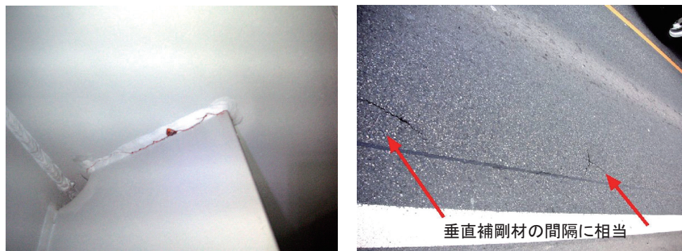
a) 鋼床版の疲労き裂
