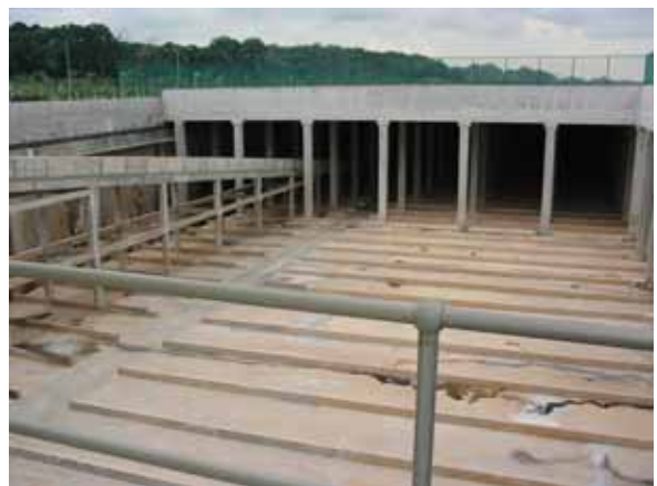
HydroSelf® flushing system in Singapore
