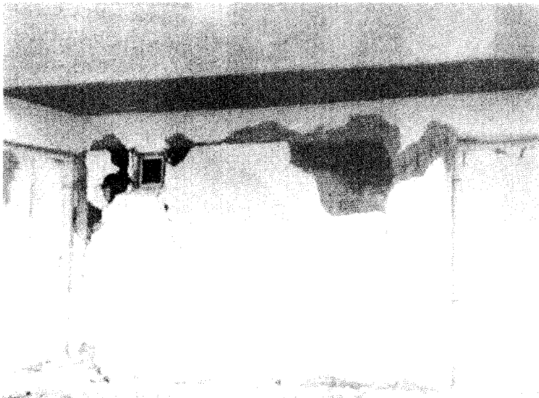
3) Big cracks, Massive Spalling of cover concrete and extensive exposure of reinforcing bars are observed.
