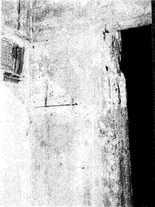
1) Big cracks, Massive Spalling of cover concrete and extensive exposure of reinforcing bars are observed. But buckling of the reinforcing bars is not observed.
