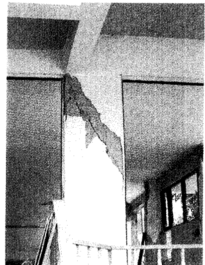
Big shear crack at the top of column
