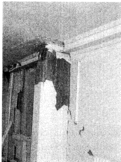
Big shear crack at the top of column
