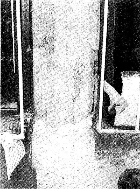
4) Corner cover concrete is spalled off. But shear cracks are not observed.
