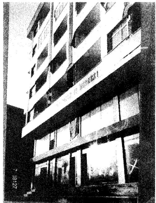
4) Rank C: Diagonal cracks observed in upper stories. Keeping out is needed near the building.
