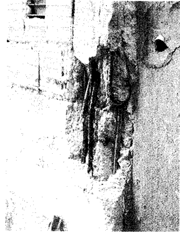
Concrete crush at the bottom of column and foundation beam-column joint.
