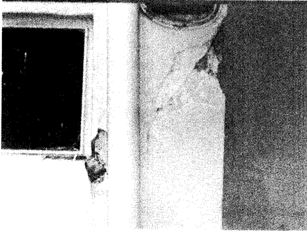
1) Wide shear cracks and local crush of cover concrete are observed at the upper part of column.
