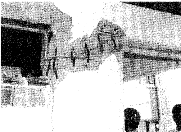
7) Buckling of reinforcing bars
