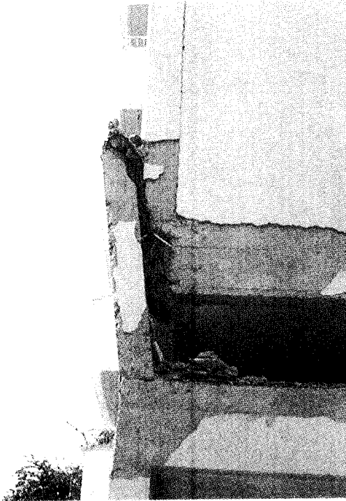
1) Visible settlement and/or inclination of floor
