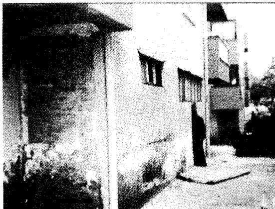
1) Rank A: Local crack and cracks at the boundary between wall and RC frame
