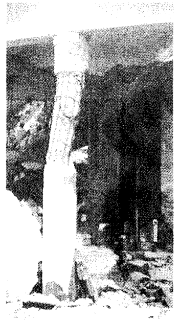
6) Crush of core concrete
