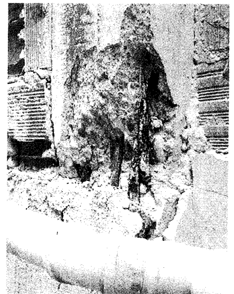
4) Local crush of cover concrete and exposure of reinforcing bars are observed. But no cracks are observed in core concrete.
