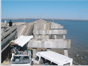
写真-3 橋梁の被災
