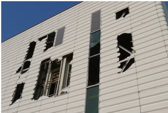
Photo 39 Breakage of exterior and windows
