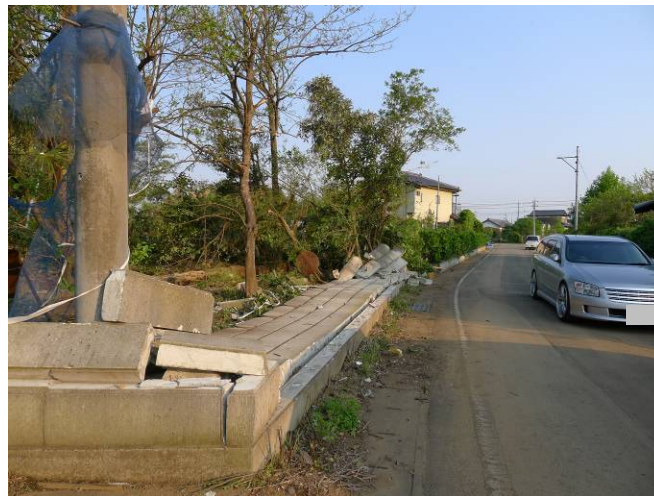
Photo 32 Collapse of stone fence
