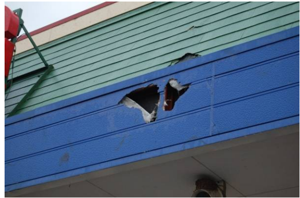
Photo 26 Evidence of collision to exterior material
