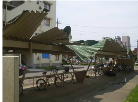
Photo 31 Heavy deformation of roof of a bicycle park
