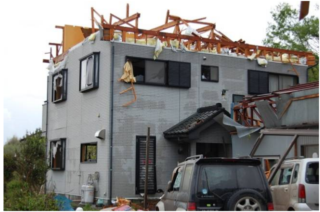
Photo 10 Wood House H whose gable roof was scattered.
