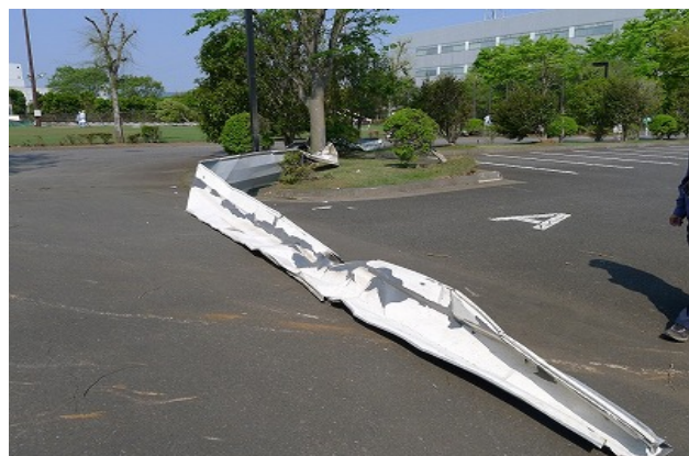
Photo 42 Scattered roofing materials
