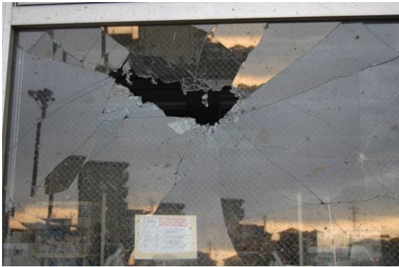
Photo 25 Evidence of collision to window
