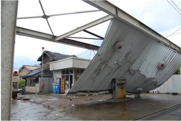
Photo 30 Collapse of a gas station roof
