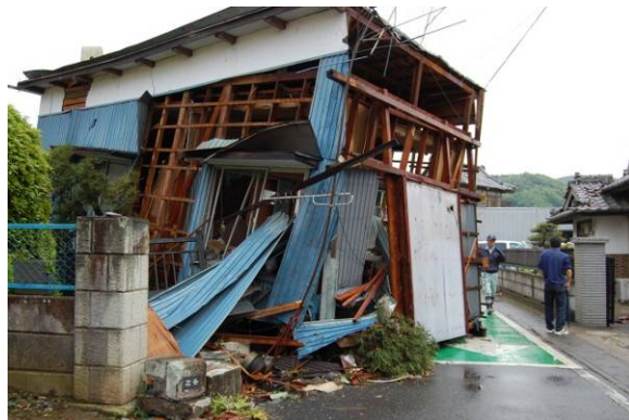
Photo 8 Wood House F which moved horizontally
