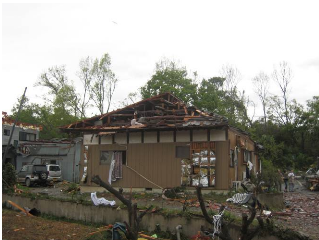
Photo 11 Wood House I whose hipped roof was scattered
