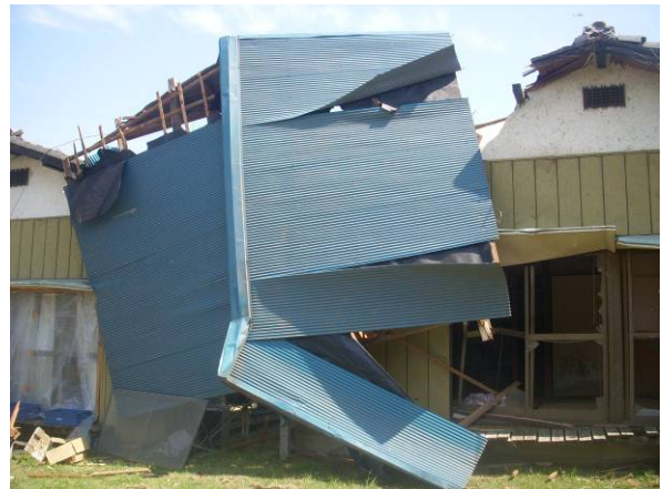
Photo 28 Collision of flying roof frame
