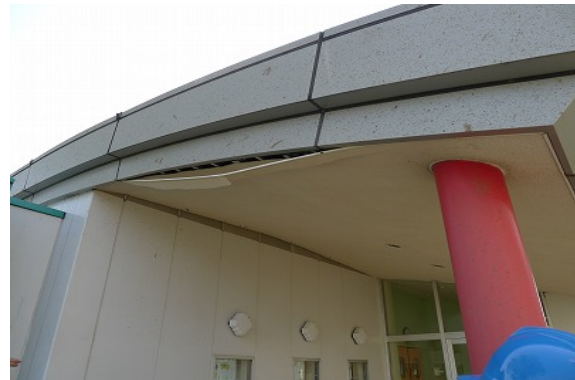
Photo 40 Breakage of eave soffits
