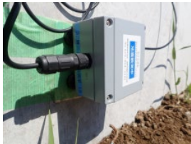
Sensor installation status
