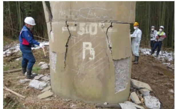
Photo 1. Edano Bridge in Kakuda City, which was damaged by an earthquake
