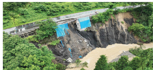
Fig. 1. Damage to National Highway 121 due to torrential rainfall in August 2022 (Yonezawa, Yamagata)
