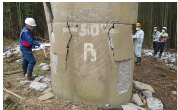
Photo 1. Edano Bridge in Kakuda City, which was damaged by an earthquake
