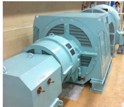
Photo 1. Management Use Electric Power Generating Equipment (Sagae Dam)
