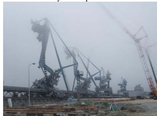
Photo 1. Collapsed Unloaders at Soma Harbor
