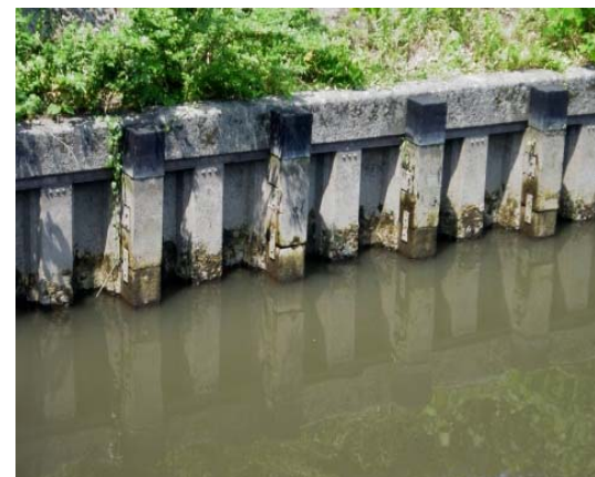
矢板護岸の腐食
