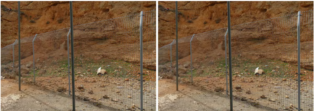
Figure 2.4-20. West-side pier and fallen debris around it
