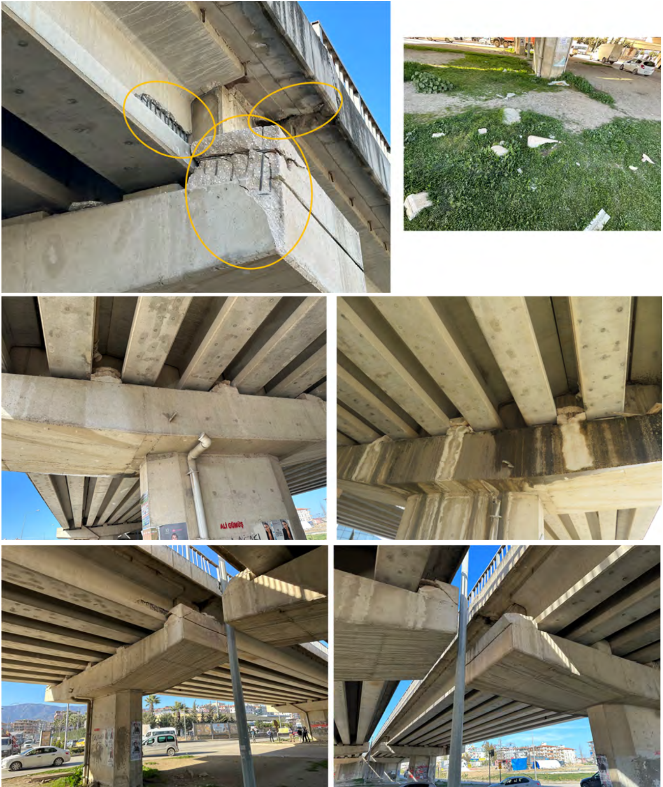
Figure 2.1-4. Examples of observed damage to girder ends and shear keys
