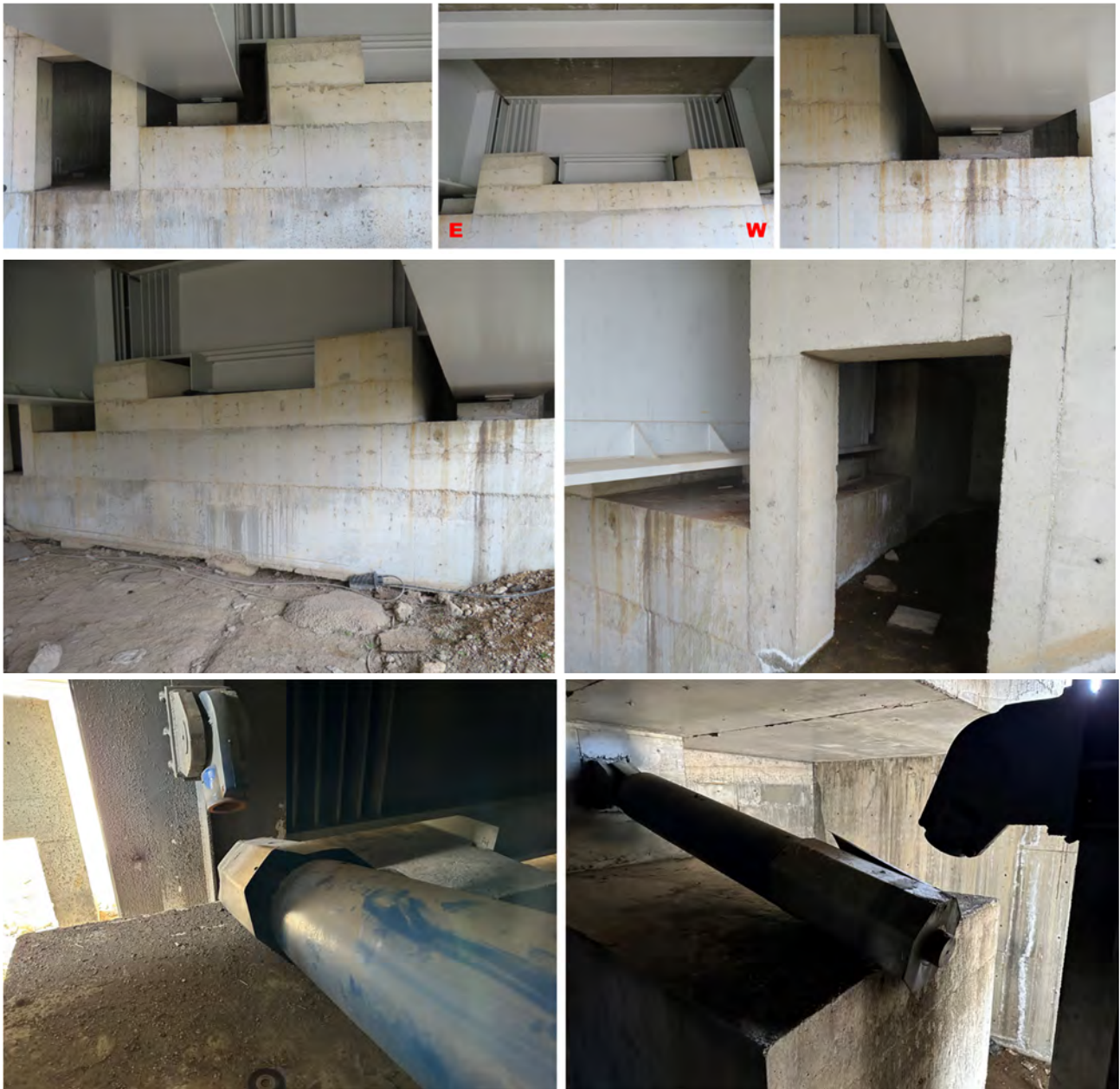
Figure 2.4-26. Damage to dampers
