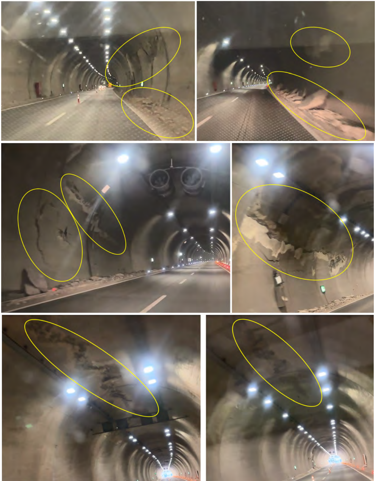
Figure 2.4-9. Examples of observed damage to Erkenek tunnel
