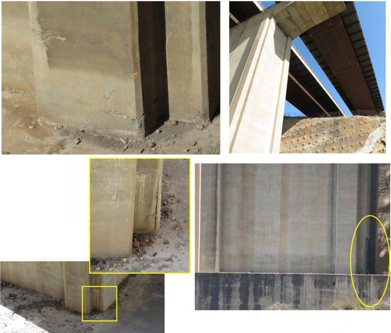
Figure 2.3-9. Examples of damage to column bases
