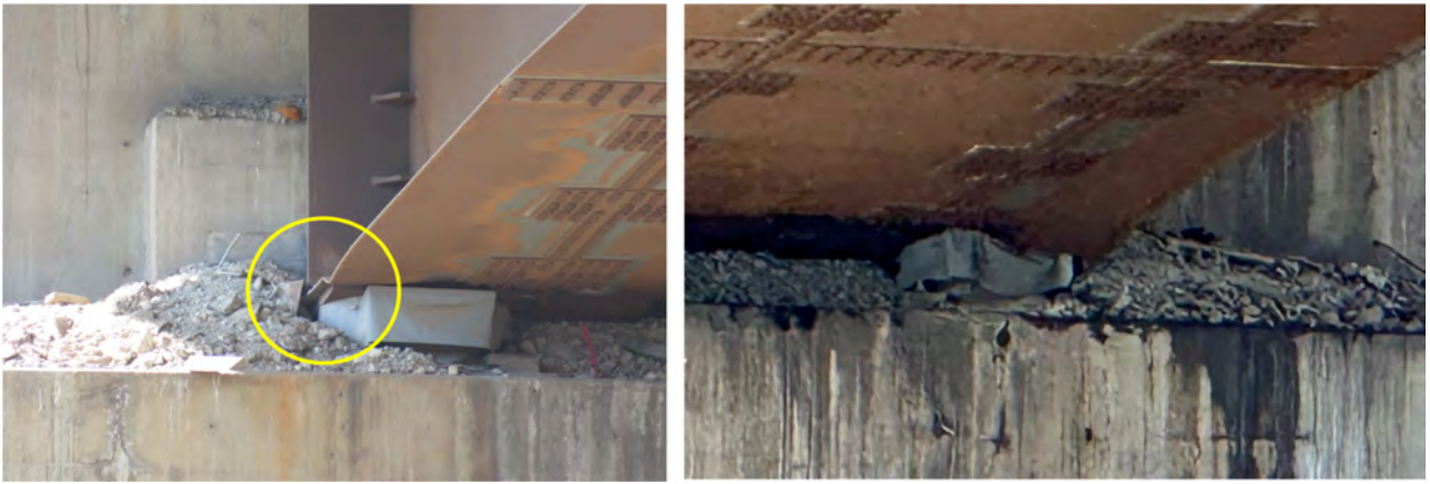
Figure 2.3-24. Local buckling of bottom flange above bearing on in-service side of bridge
