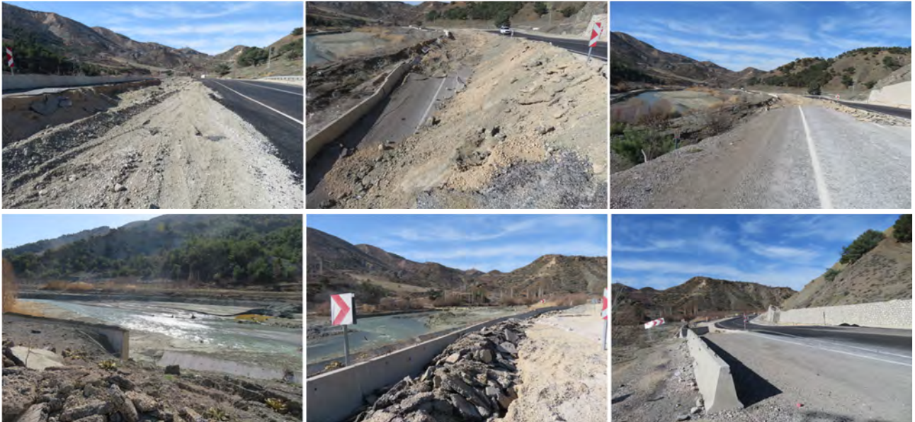
Figure 2.4-3. Examples of observed damage to road embankments
