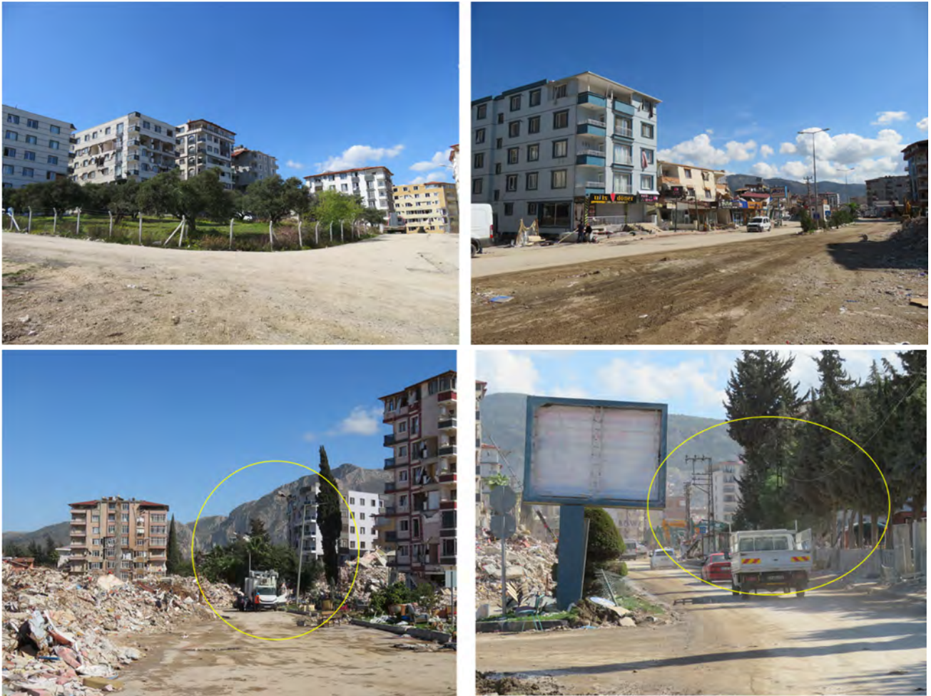
Figure 2.5-1. Examples of observed damage to buildings and road ancillaries in downtown Antakya city
