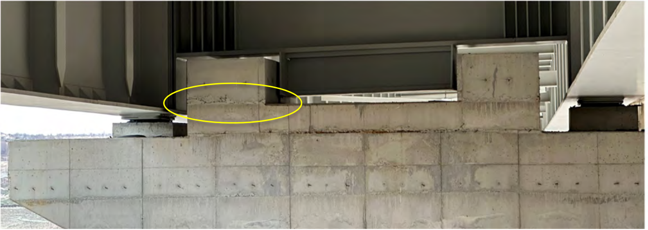
Figure 2.4-31. Damage to shear keys on pier of new bridge
