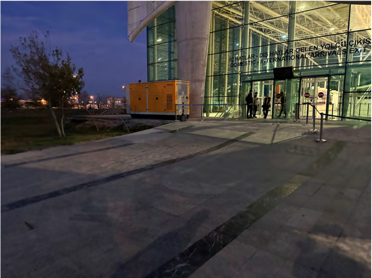
Figure 2.1-21. Slumping of ground surrounding Hatay Airport Terminal building
