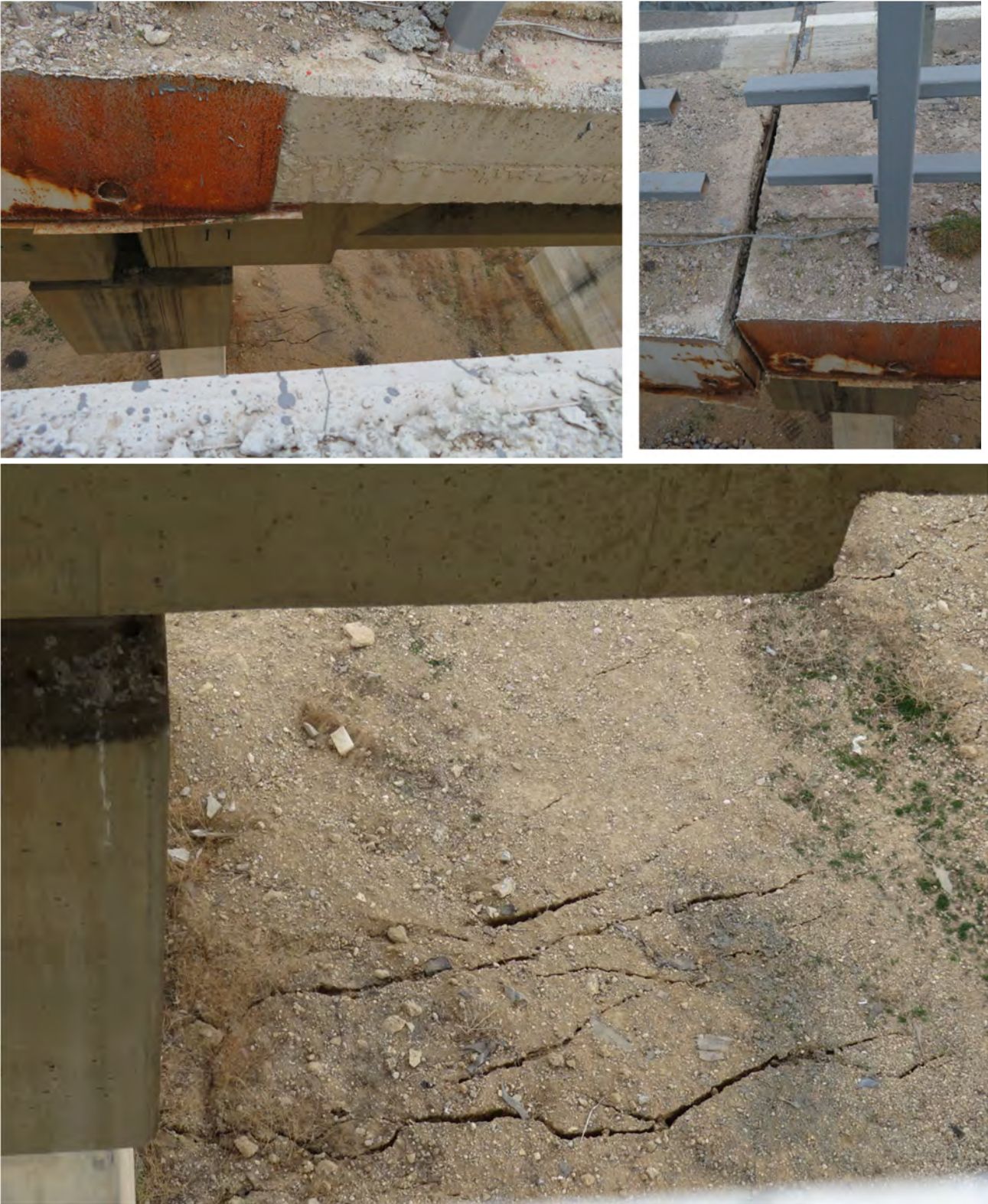
Figure 2.4-33. Dislocation of spans from each other over piers and cracks on ground surface
