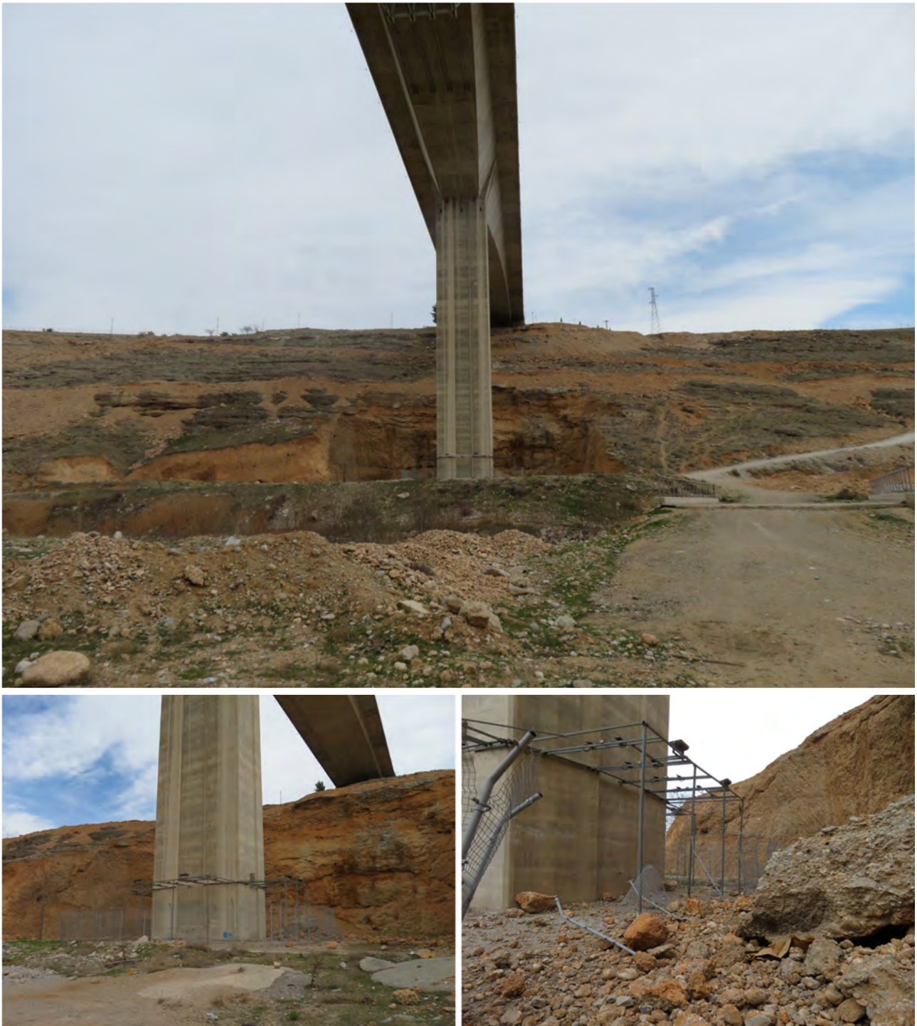
Figure 2.4-18. East-side pier and fallen rocks
