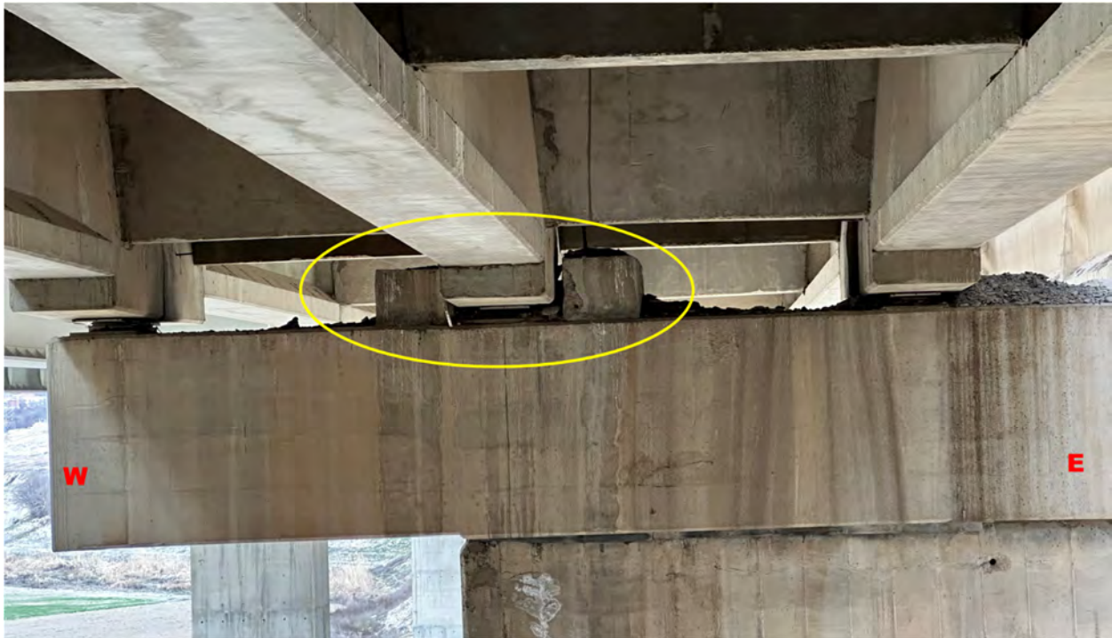
Figure 2.4-30. Damage to shear keys on pier of old bridge
