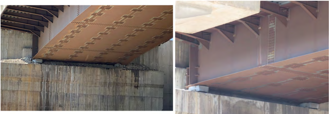
Figure 2.3-23. Abutments on Osmaniye side: Left = in-service side of bridge, Right = closed side of bridge
