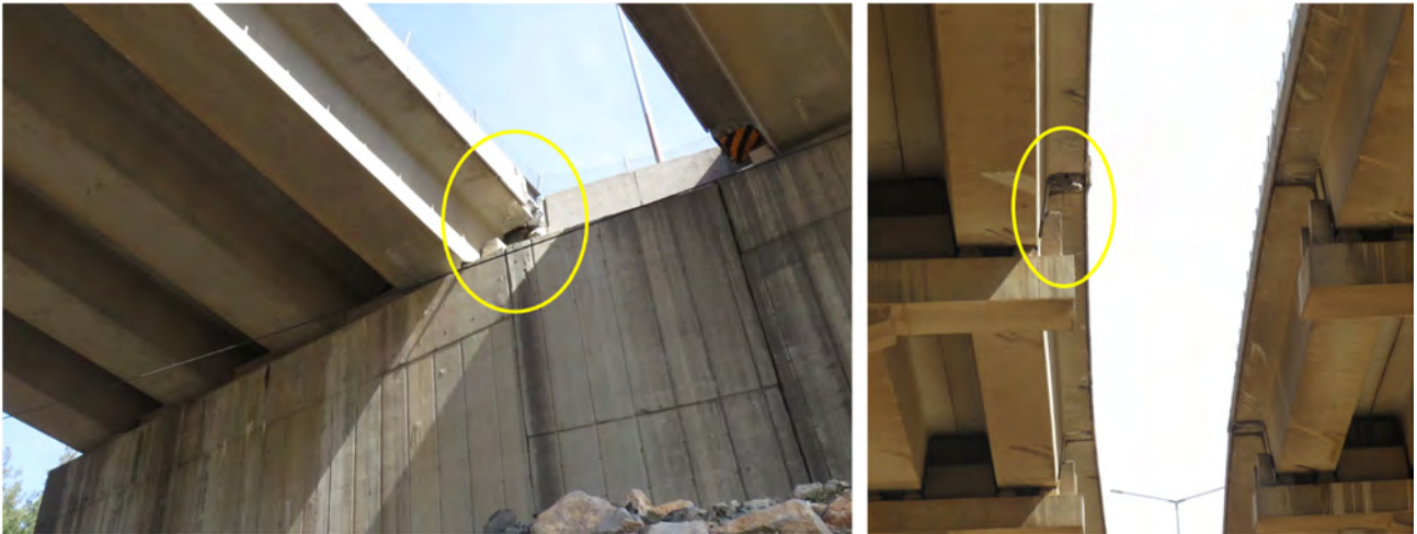
Figure 2.3-29. Examples of damage to expansion joint and link slabs
