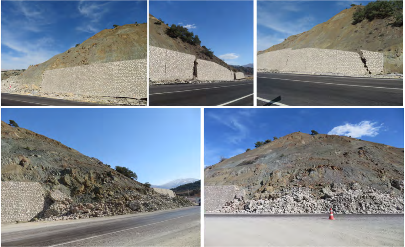
Figure 2.4-5. Cut-slope failure with collapse of retaining wall
