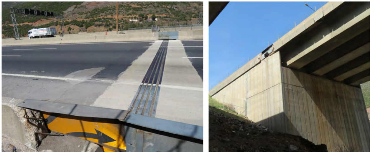
Figure 2.3-37. Deformed plates in transition section of parapet walls between bridge and backfill sections
