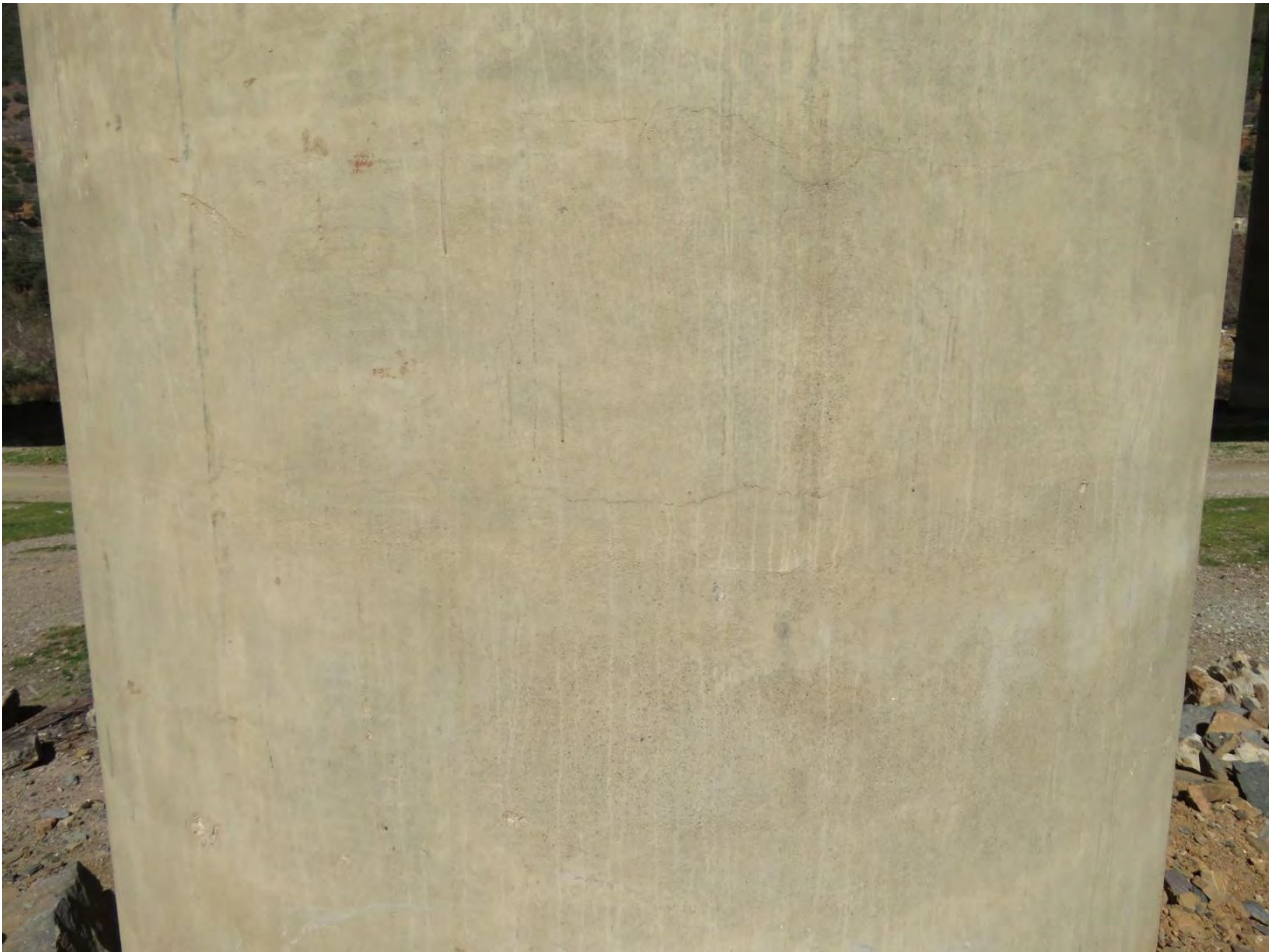
Figure 2.3-39. Horizontal crack in column
