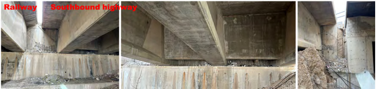
Figure 2.4-29. Examples of damage to abutment parapet wall and shear keys
