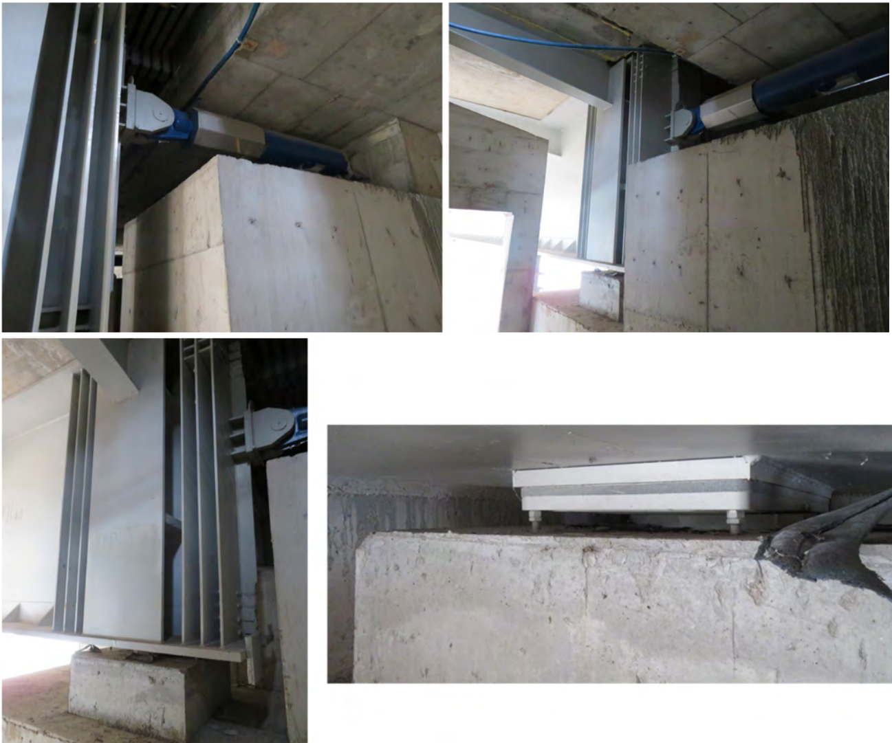
Figure 2.4-36. Dampers and bearings in north-side abutment of new bridge
