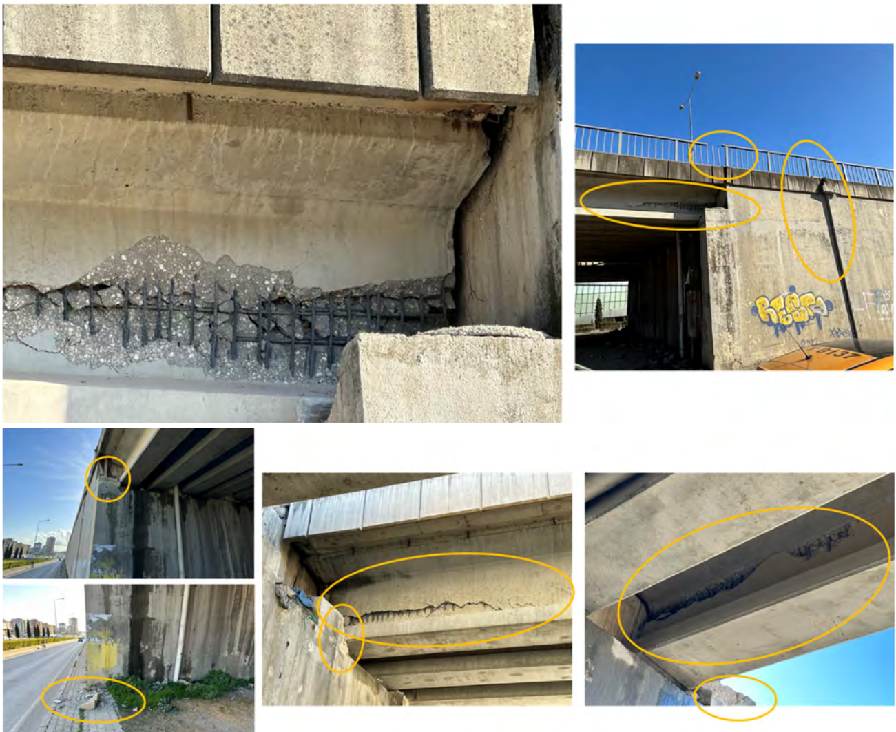
Figure 2.1-3. Damage to girder ends and shear keys
