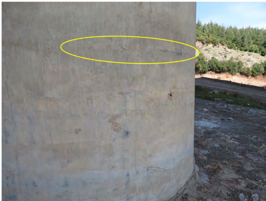
Figure 2.3-28. Horizontal crack in bridge column
