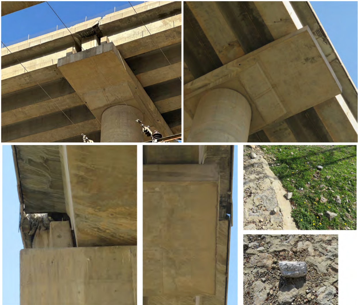
Figure 2.3-4. Damage to link slabs
