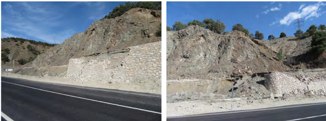
Figure 2.4-4. Damage to retaining walls
