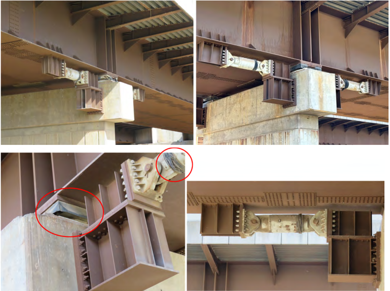
Figure 2.3-43. Dampers of Vecdi Diker viaduct
