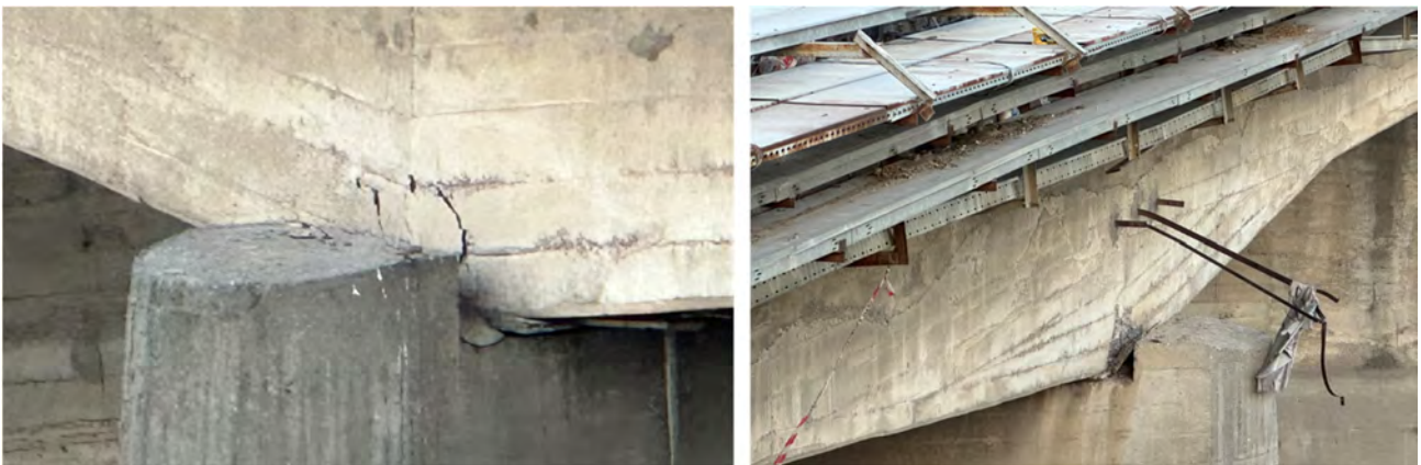
Figure 2.1-14. Example of damage to Bridge #4
