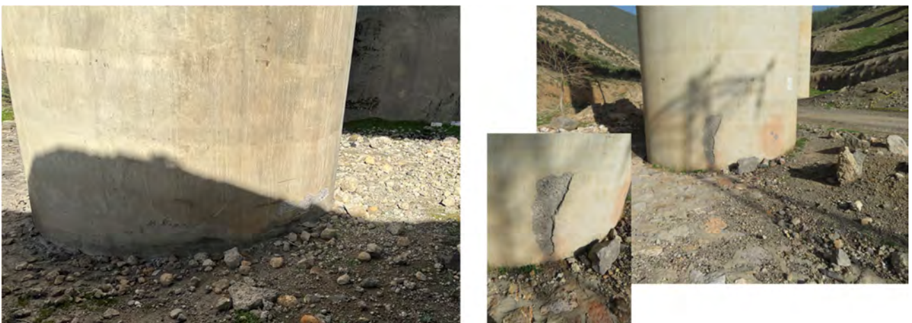
Figure 2.3-5. Examples of damage to columns
