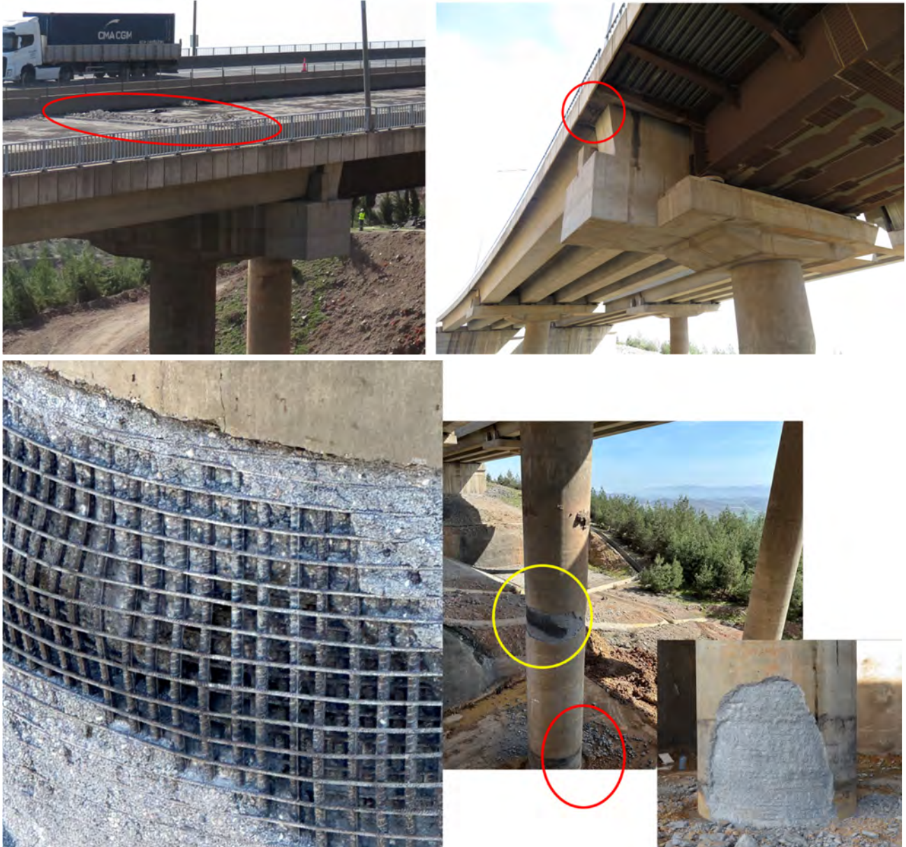
Figure 2.3-21. Severe damage to column supporting transition section from concrete girder to steel-box girder on closed side of bridge
