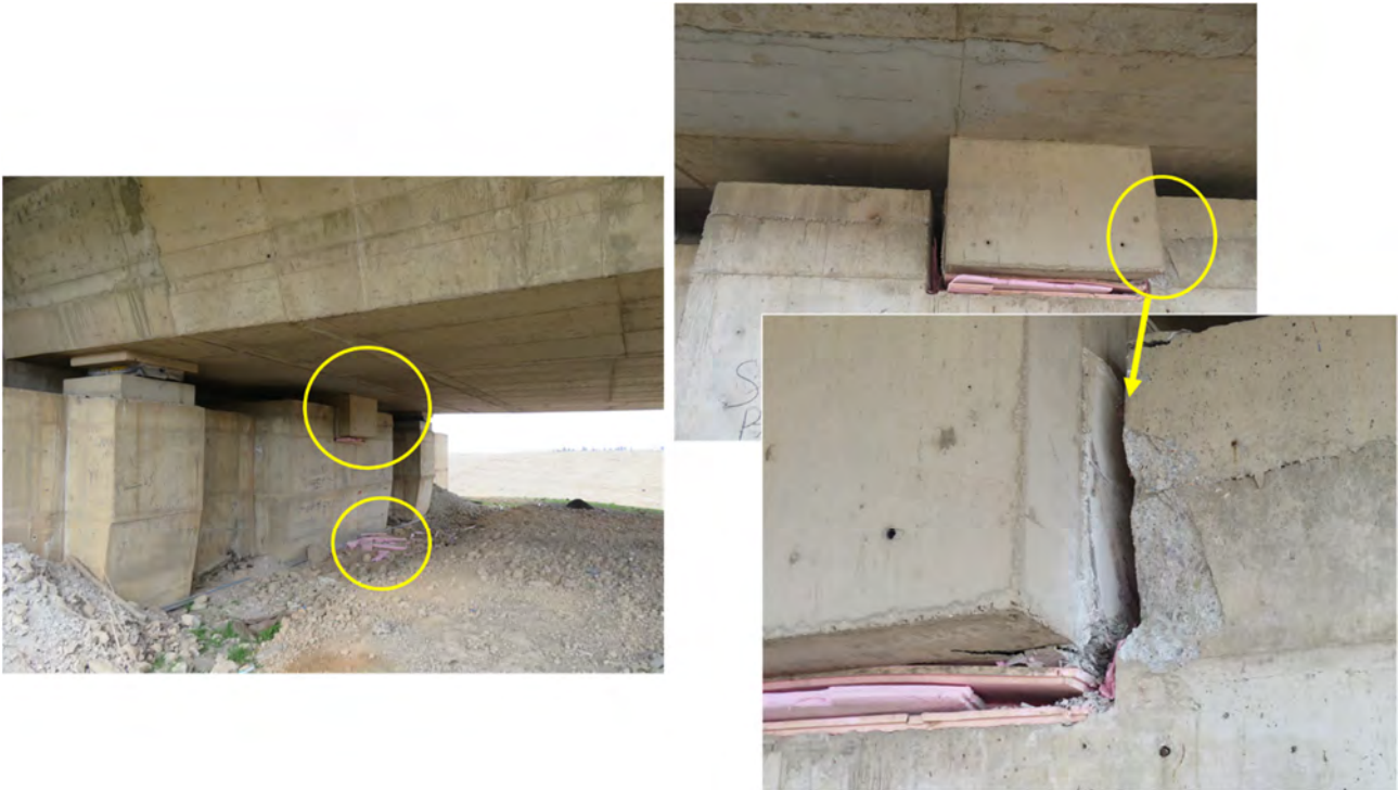
Figure 2.4-16. Examples of observed damage to shear key on west-side abutment.
