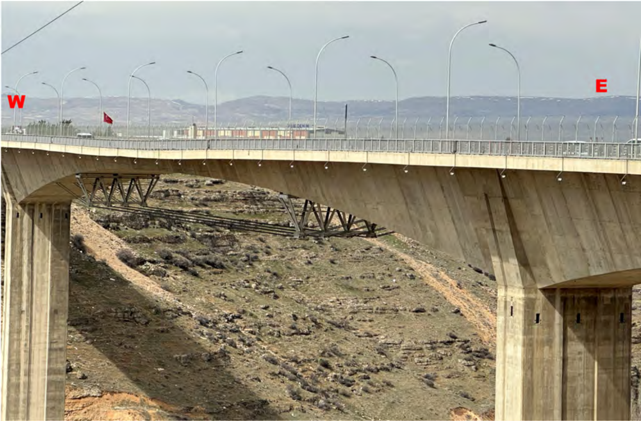
Figure 2.4-13. Center span sagging and outer cable system
