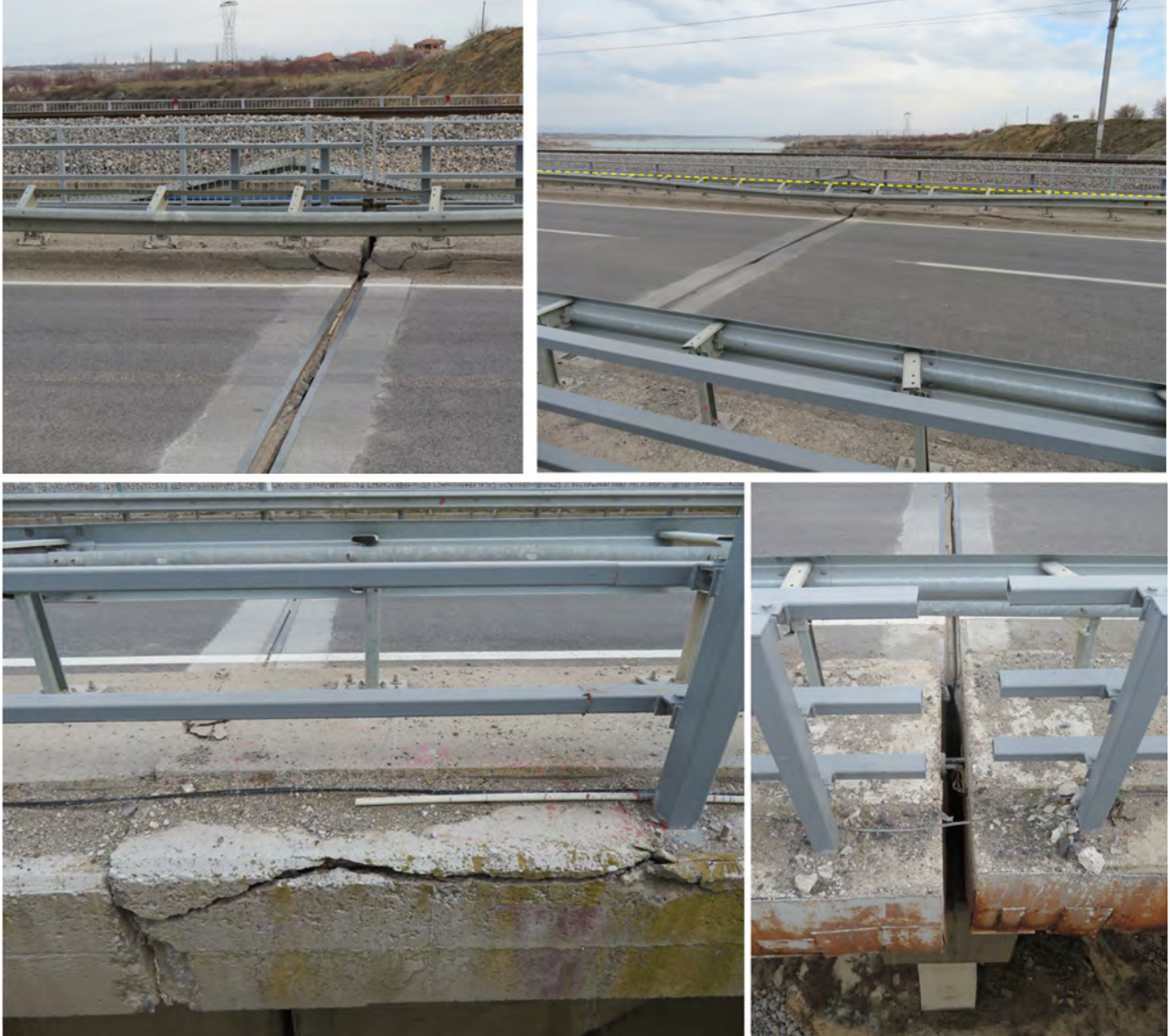
Figure 2.4-32. Dislocation of spans from each other over piers
