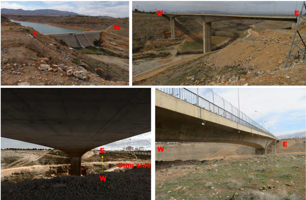
Figure 2.4-12. Beylerderesi Turgut Özal viaduct on D850 (E and W denote the east and west sides of bridge, respectively, in photos)
