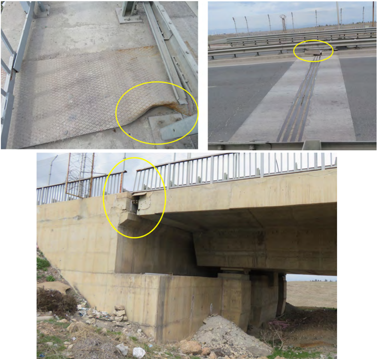
Figure 2.4-15. Examples of observed damage to girder-end and west-side abutment
