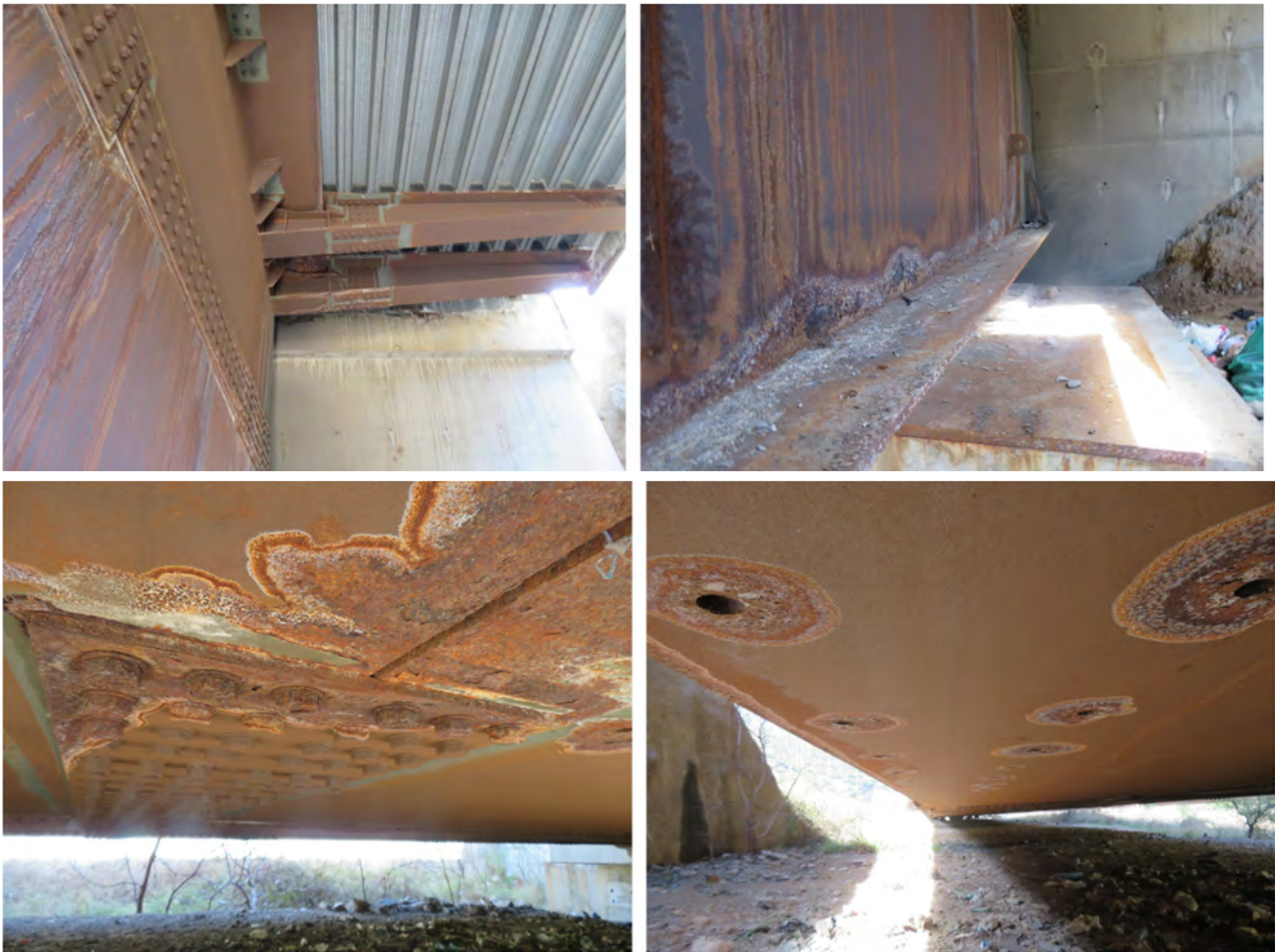
Figure 2.3-34. Nonuniform rust development in weathering steel girder
