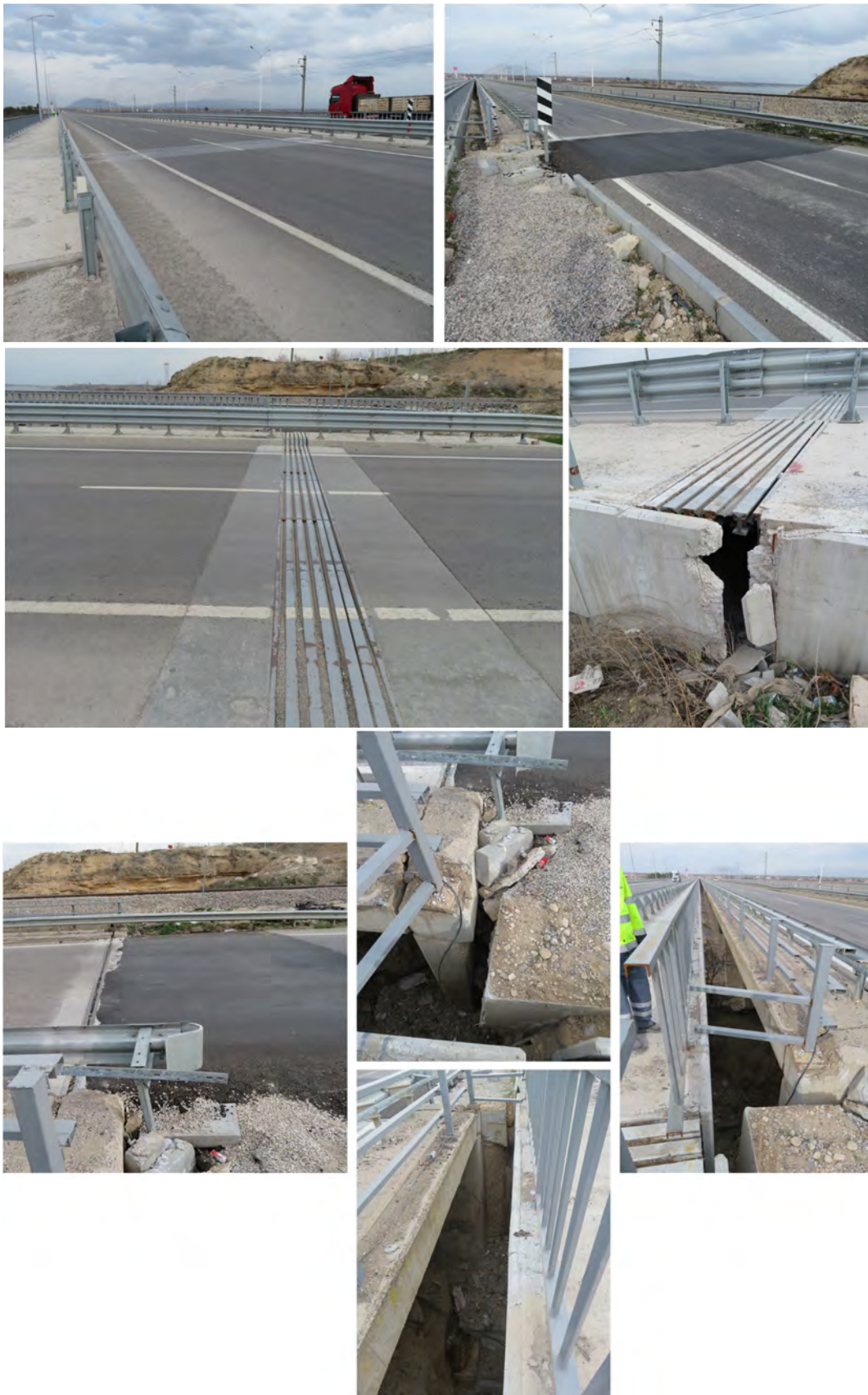
Figure 2.4-25. Examples of damage around south-side abutment
