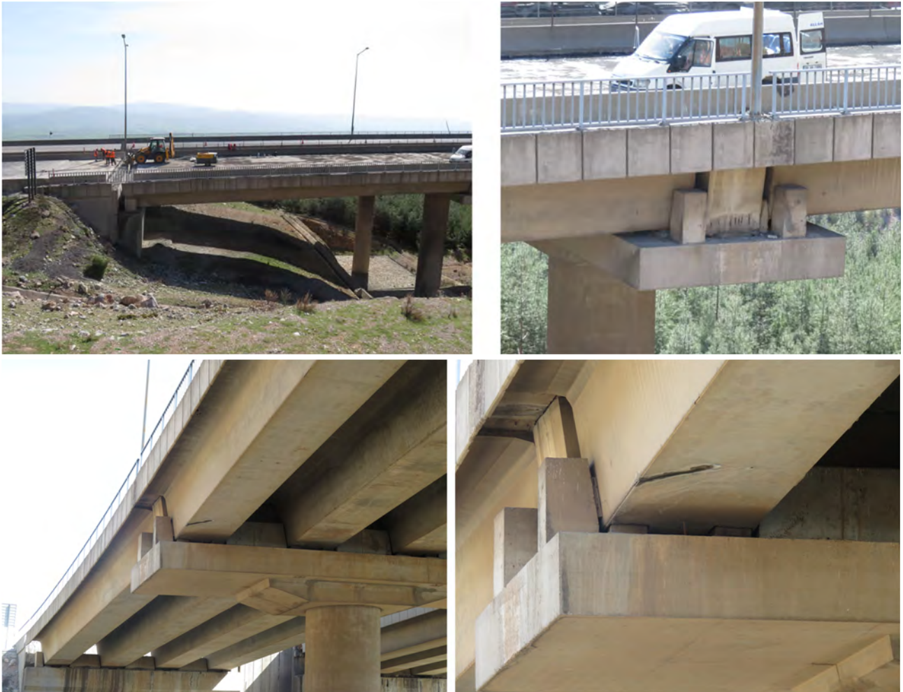
Figure 2.3-20. Expansion joint replacement work on Gaziantep-side abutment and concrete block to support link slab on column next to abutment on closed side of bridge.
