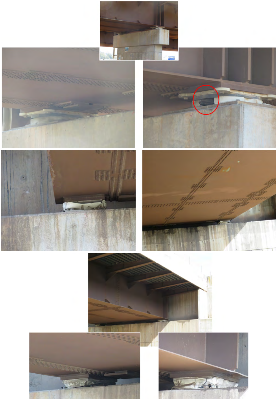
Figure 2.3-44. Examples of observed damage to bearing covers
