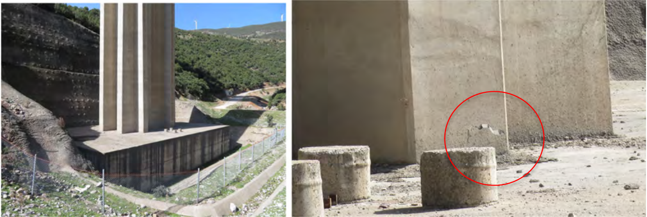
Figure 2.3-16. Examples of damage to column bases
