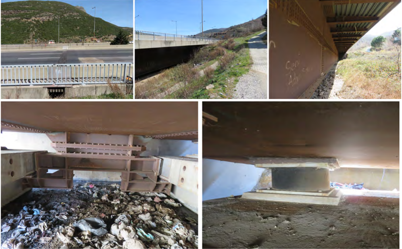
Figure 2.3-33. Photographs of expansion joint, bearing, and lateral displacement restrainer on Gaziantep-side abutment on mountain-side bridge
