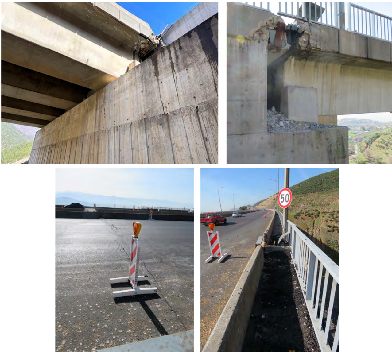
Figure 2.3-6. Examples of damage due to collision of superstructure and abutment at Gaziantep side
