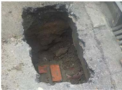
O市: 取付管、取付管接合部破損、長さ1.2×幅0.8×深さ0.7m
