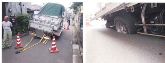
S市: 150mm (取付管)、S47、接合不良、長さ0.5×幅0.4×深さ0.5m
