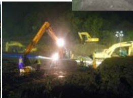
Digging of temporary drainage channel conducted 24hrs per day between June 18th and 26th
