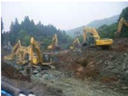
Measures commenced on June 17th to relieve blockage (natural dam)
