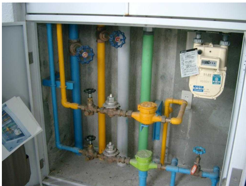
Photo 1 - Example of distinction by color-coding the pipes (Yellow is reclaimed wastewater, blue is drinking water)
