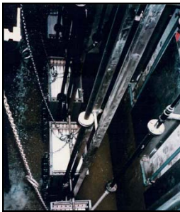
Membrane modules placed in tanks
