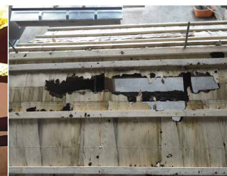
Photo 2 Example of fire burning through roof underlayer
