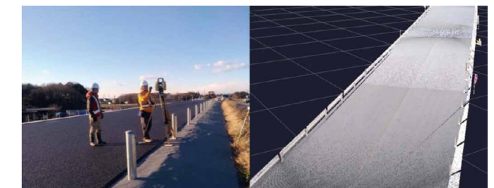
Figure. Completed work measurements using a laser scanner (left) and acquired point group data (right)
