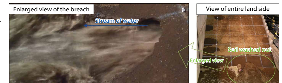
Photo: View of sudden breaching
