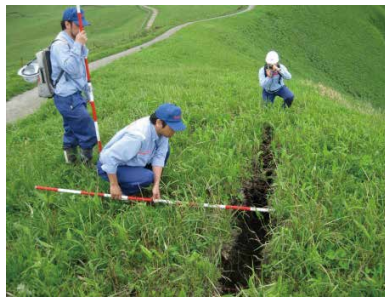
Photo 1. Surveying cracking caused by the earthquake
