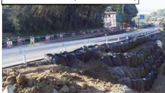
Photo Technical guidance with emergency restoration (From a Road Bureau press release)
