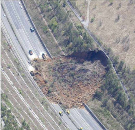
② Oita Expressway (impassable)
