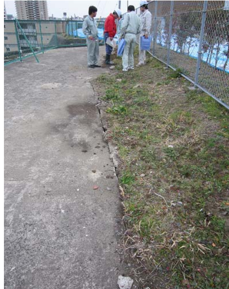
Photo 3.3.1.3 A crack is seen in a parking area
