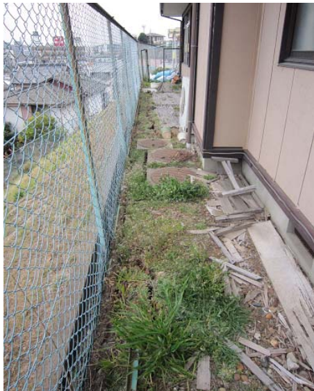
Photo 3.3.1.2 A crack is seen
