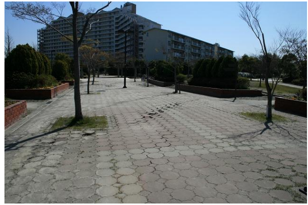
(b) Ground unevenness on the park road
