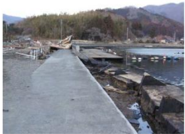
(b) Seawalls collapsed to seaside (Nagahama district, coastal protection area in Ofunato Port) (Crown height of walls T.P. + 3.00m, Observed tsunami trace height T.P. + 10.02m)
