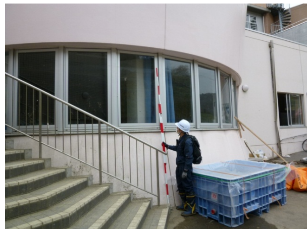
Photo 3.3.1.20 A flood trace (at the top of the pole) at the elderly welfare center
