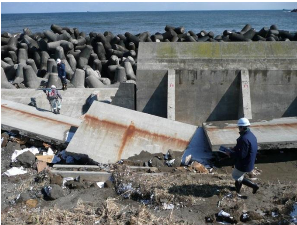
(a) Collapsed seawalls in Ichikawa district, Hachinohe Port
