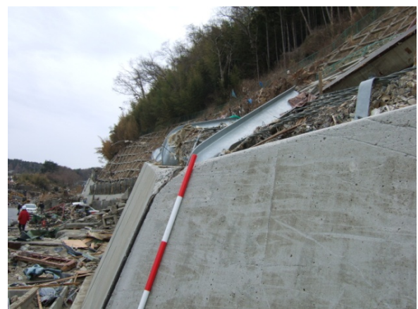
Photo 3.3.1.15 Scratch marks on the retaining wall
