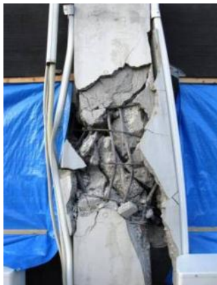
Photo 3.3.9.1 Shear failure of short column
