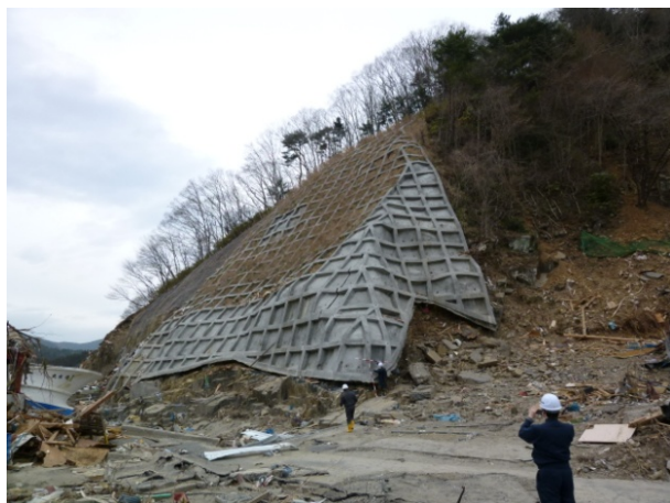
Photo 3.3.1.12 Cribwork leg portion washed away (Kawajiri area)
