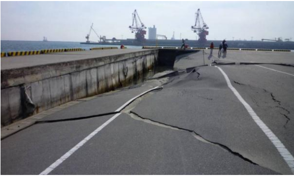
Photo 3.3.7.3 Sunken wharf apron at Onahama Port
