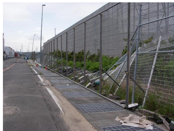
(a) Damage of fence (North pier section of Minato-district, Hitachinaka Port Area, Ibaraki Port, drifted containers were removed) (Crown height of walls T.P. + 2.20m, Observed tsunami height T.P. + 4.32m)
