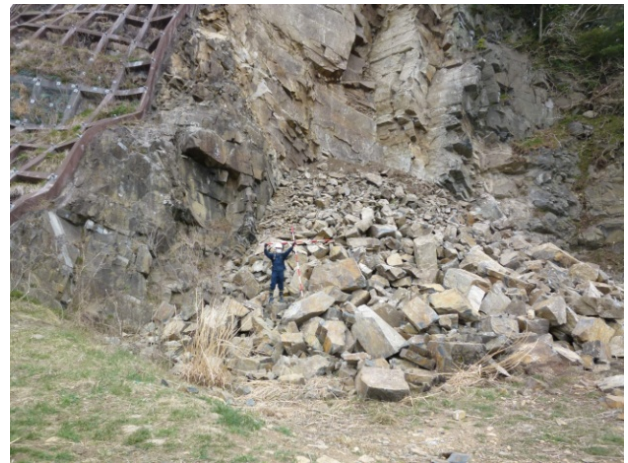
Photo 3.3.1.9 Earth falls on the right side of the cribwork (Ishinomaki)
