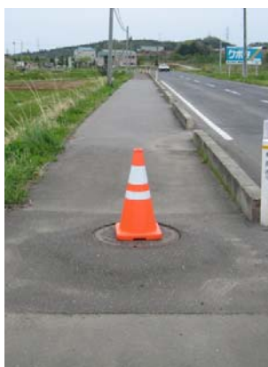
Photo 3.3.2.7 A portion subjected to the anti-liquefaction measure (damaged part)
