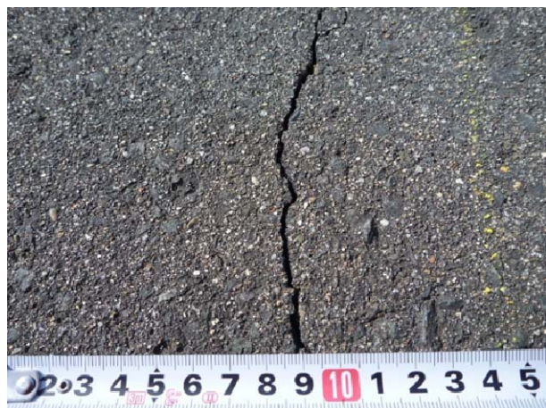
Photo 3.3.4.2 Close-up of a crack that appeared on the dam crest pavement (Surikamigawa dam)
