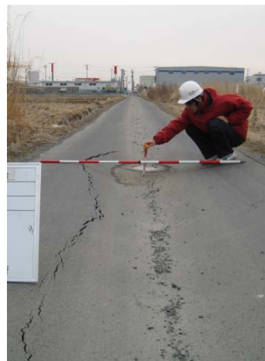
Photo 3.3.2.5 Construction subjected to the anti-liquefaction measure (slight damage)
