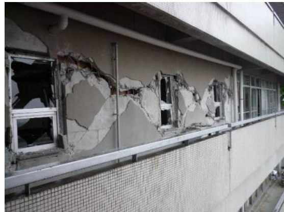
Photo 3.3.9.2 Shear failure of non-structural wall
