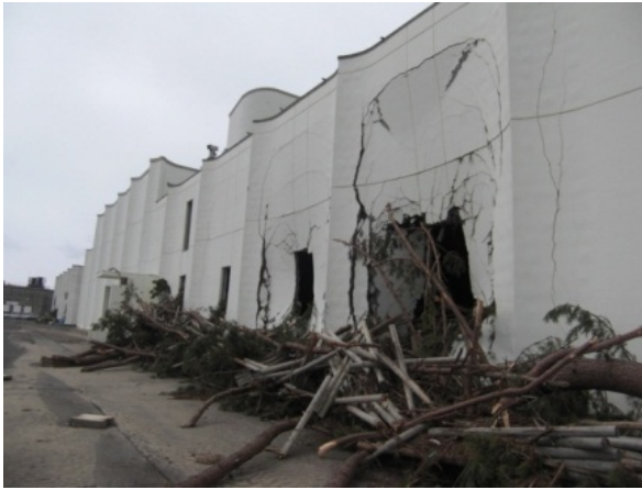
(b) Castaways' direct damage to a building
