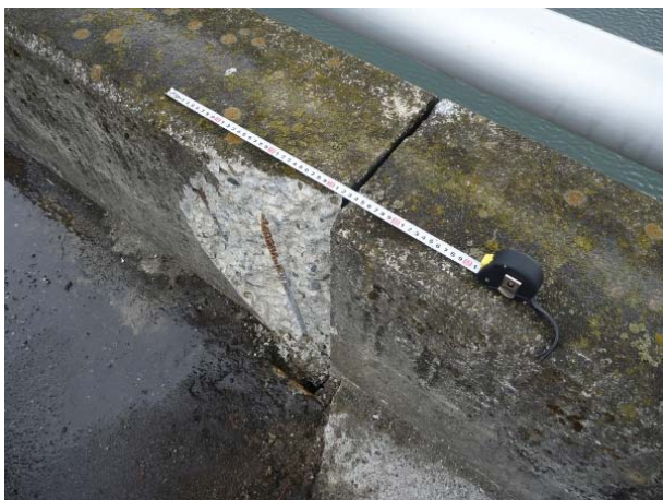
Photo 3.3.4.5 Exfoliation of parapet concrete (Tase dam)
