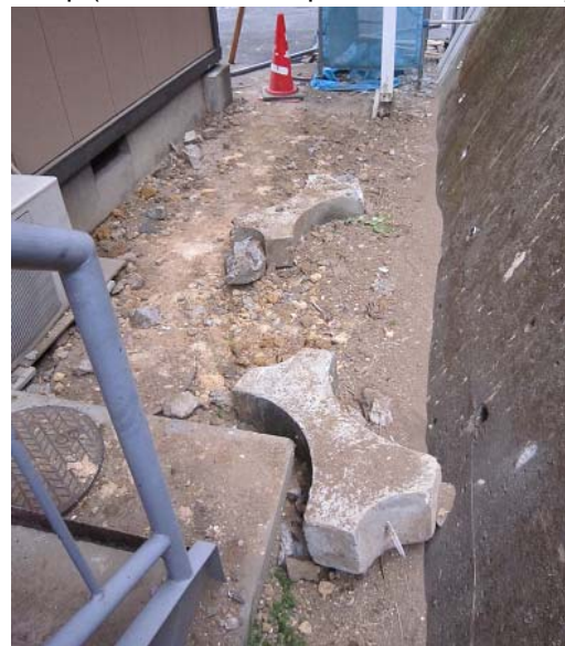
Photo 3.3.1.5 Broken cribwork pieces that dropped to the lower portion of the slope
