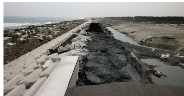
Photo 3.3.5.1 Partially Collapsed Three-Surface Armored Coastal Dike and Scouring Situation at the Landward Slope Toe (Kabasaki Coast, Iwanuma City, Miyagi Prefecture)
