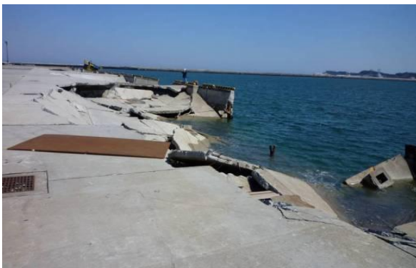
Photo 3.3.7.4 Collapsed wharf at Soma Port
