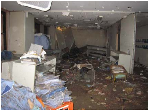
(c) Flooding-caused damage to interior equipment Photo 3.3.2.2 Representative Tsunami-caused Damage to Sewage Treatment Plants and Pumping Stations
