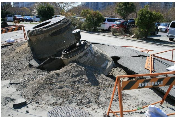
Photo 3.3.12.4 Surfacing of a water tank by ground liquefaction (Urayasu City)
