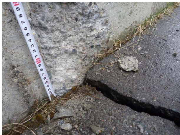
Photo 3.3.4.6 Level difference at joint of crest pavement (Tase dam)
