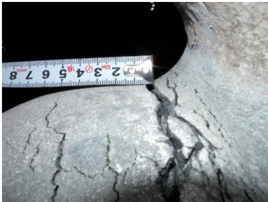
Photo 3.3.9.5 Cracks in lead damper
