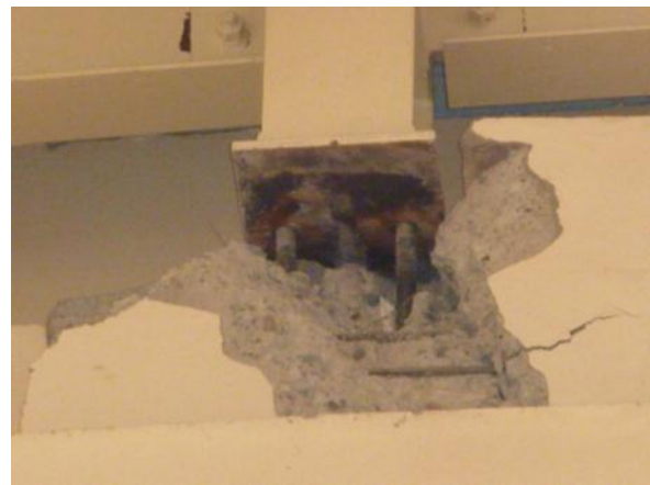
Photo 3.3.9.3 Example of damage at RC column and Steel roof joints (bearing support parts)
