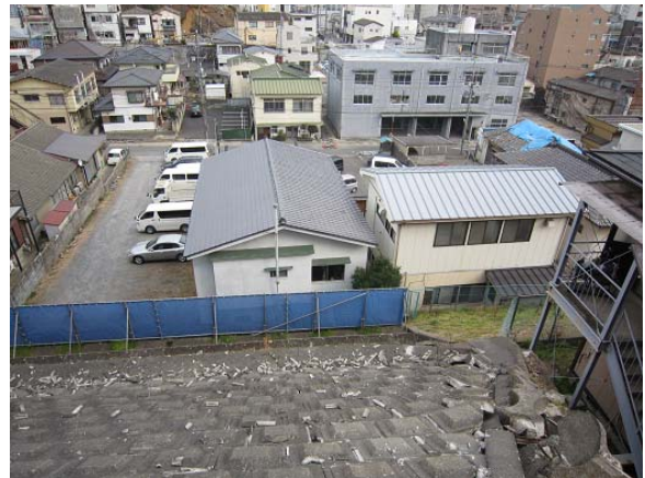
Photo 3.3.1.4 The slope's lower portion as seen from its top (broken cribwork pieces are scattered)
