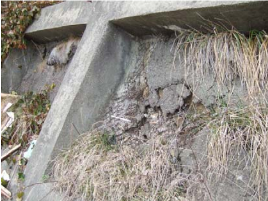
Photo 3.3.1.16 Sprayed materials are broken away from the lath
