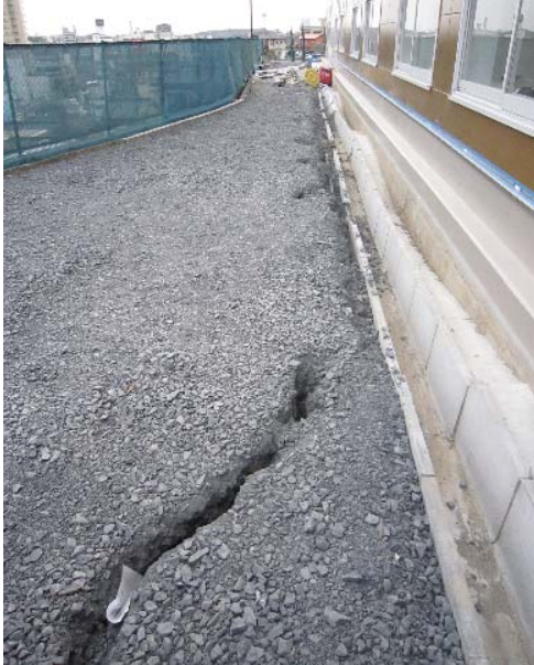
Photo 3.3.1.1 A crack along a building
