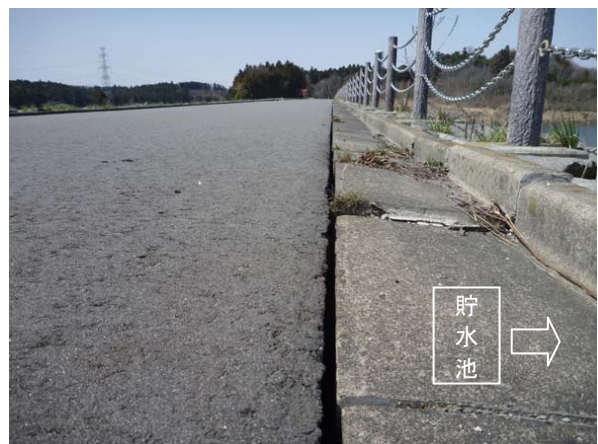
Photo 3.3.4.9 Opening between curb at the crest center and pavement (Kejonuma dam)
