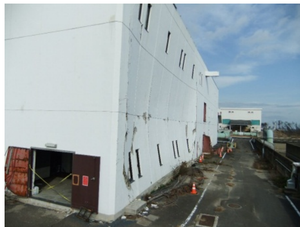
(a) Wave pressure-caused damage to a sea-side wall
