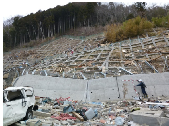
Photo 3.3.1.14 Stone guard buckling
