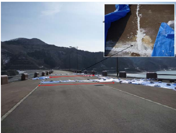
Photo: 3.3.4.1 A crack at the attaching portion of the left bank of the dam crest (Surikamigawa dam)
