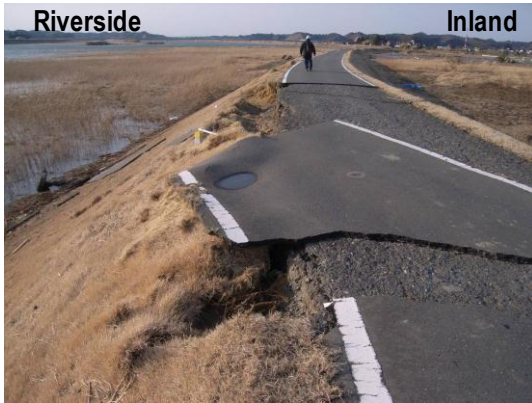
Photo 3.2.2.2 Detachment of Asphalt Paving at the Crest of the Levee (near the left bank of the Naruse River, 1kp)
