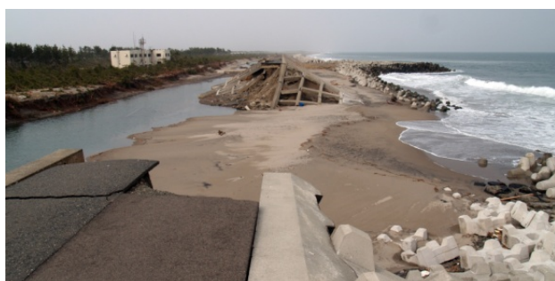
Photo 3.3.5.2 Completely Collapsed Coastal Dike (Ninokura Coast, Iwanuma City, Miyagi Prefecture)
