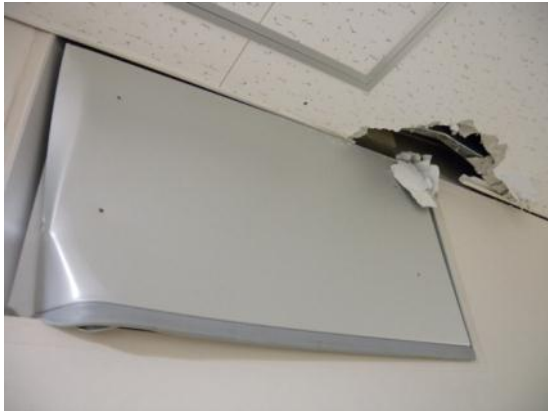
Photo 3.3.9.4 Cover broken by contact etc.
