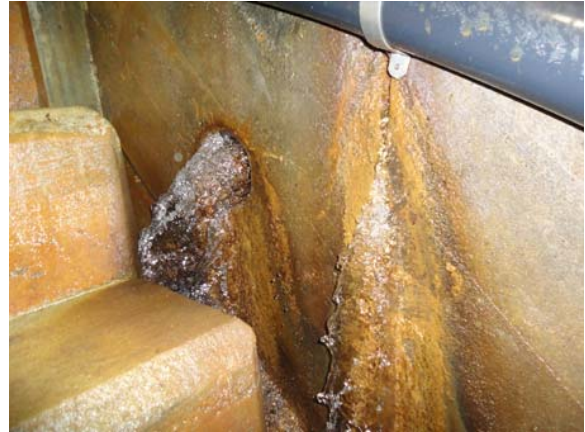
Photo 3.3.4.11 Leakage from the transverse joint (J9) (Takasaka dam)
