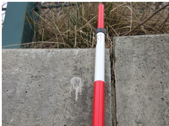
Photo 3.3.1.11 A dip slip of the retaining wall (zoomed)
