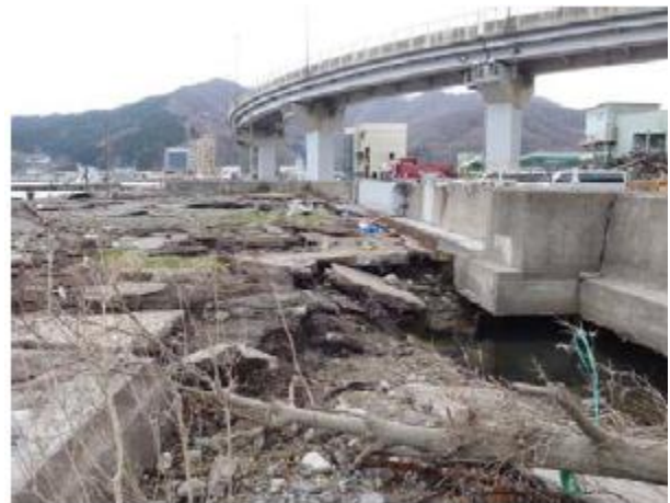
(c) Scouring observed on seaside (Suga district, coastal protection area in Kamaishi port) (Crown height of walls T.P. + 4.00m, Observed tsunami trace height T.P. + 8.64m) Photos 3.3.7.9 Tsunami damage to coastal protection facilities
