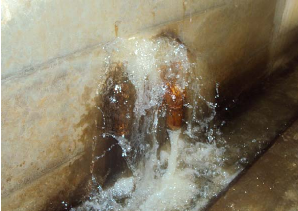
Photo 3.3.4.10 Leakage from the transverse joint (2J3) (Kamuro dam)
