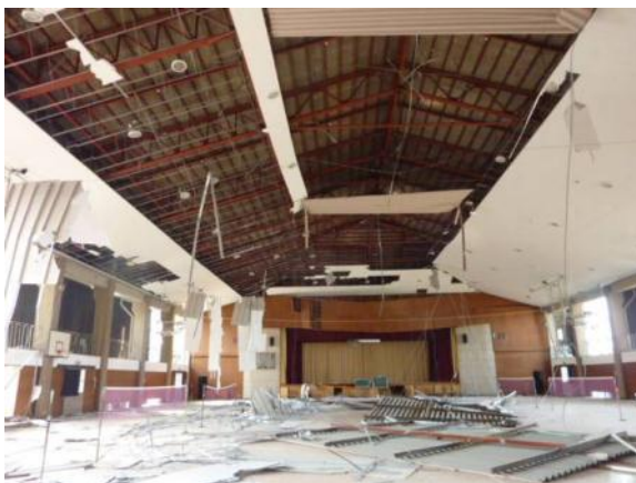
Photo 3.3.9.6 Collapse of furring ceiling
