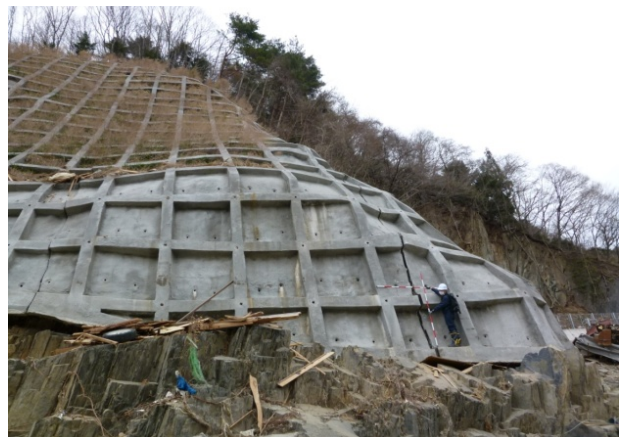
Photo 3.3.1.13 A crack at a cribwork construction joint
