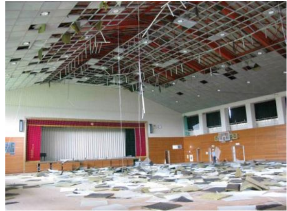
Photo 3.3.9.7 Collapse of integrated ceiling
