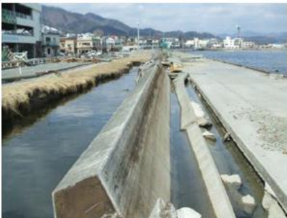
(a) Seawalls collapsed to landside (Chayamae district, coastal protection area in Ofunato Port) (Crown height of walls T.P. + 3.40m, Observed tsunami trace height T.P. + 8.07m)
