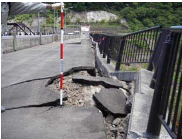
Photo 3.3.4.3 Crest of the Ishibuchi dam (earthquake of 2008)
