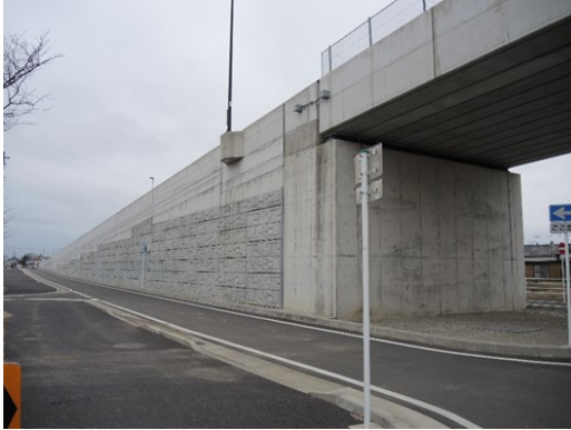
Photo 2: Example of earthwork structure with new form (abutment back approach part with reinforcing clay wall)
