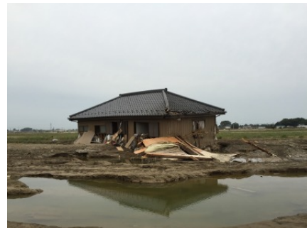
Photo 1. Wooden residential house whose structural frame was heavily damaged and washed away
