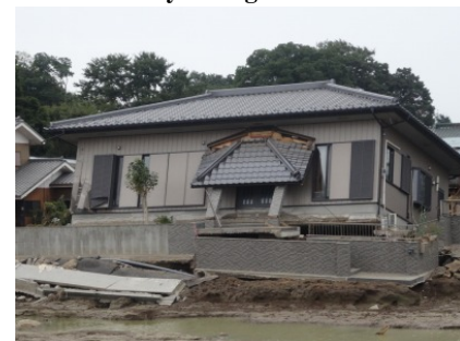
Photo 2. Wooden residential house with the ground of its premises scoured
