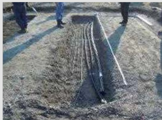
Photo 1: Checking damage to underground cables
