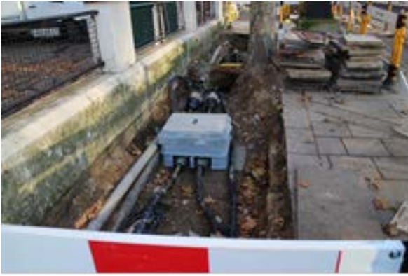
Photo 2: underground cables in London
