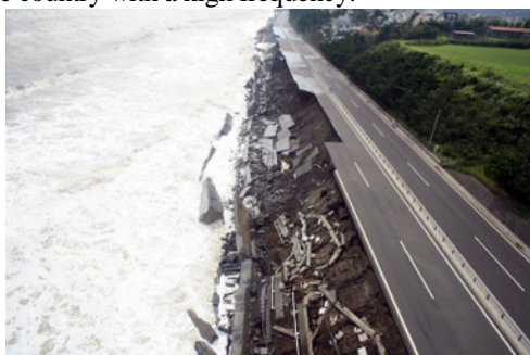
Photo: Damage to Seisho Bypass in 2007 (Source: Homepage of Yokohama River and National Highway Office, Kanto Regional Development Bureau)
