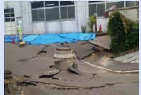
Manhole floating from liquefaction
