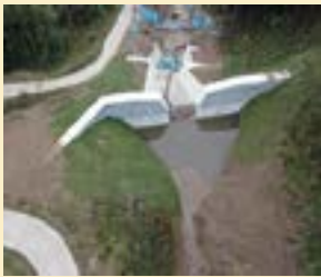
Construction of a Sabo dam with high capture capacity of sediment and driftwood trapping performance (Suzaka City, Nagano Prefecture)
