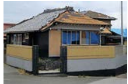
Example of damage to tile roofs caused by a typhoon (Typhoon Faxai in 2019)
