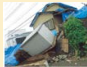
Damaged residential lots and housing
