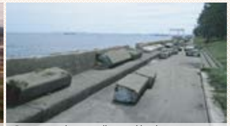
Damage to the seawall caused by the storm waves of Typhoon Faxai in 2019
